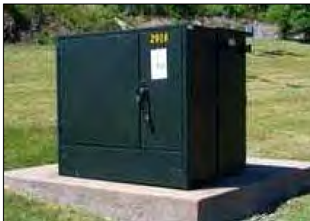
Figure 24: Pad-Mounted Distribution Transformer
