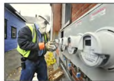
Zach Pomeroy, wearing face and hand safety equipment, installs new smart meters at homes on Brackett Street in Portland. John Ewing/Staff Photographer
